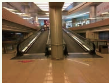
华润五彩城电梯变频改造项目 Variable-frequency escalator upgrades in Beijing Hi5
