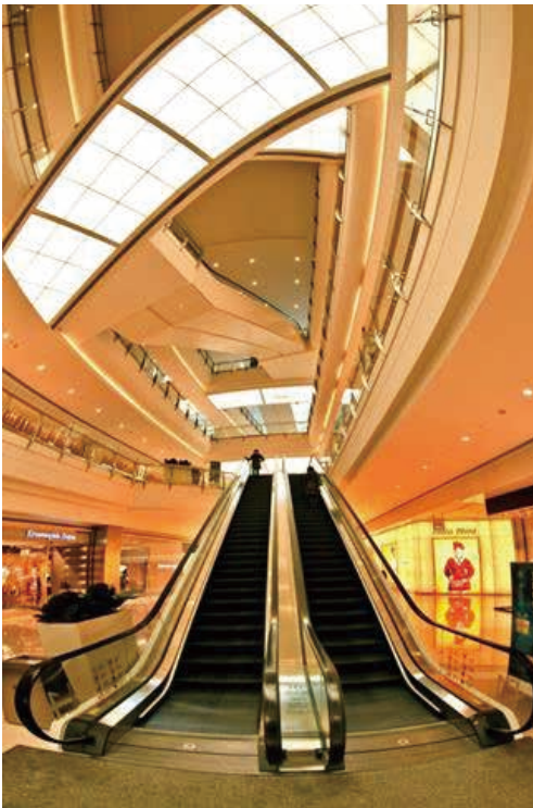
沈阳万象城中庭竖向变风量技术应用 Application of vertical variable air rate technology for the mall atrium in The MIXC (SHENYANG)
